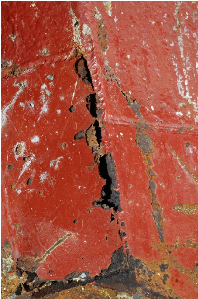
Photo 2: Damage to lower part of a corrugated bulk head. Note severe corrosion in way of areas with damaged paint.
