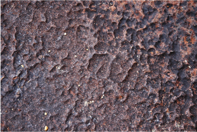
Photo 1: Damage to tank top due to corrosion caused by wet sulphur. Note the steep sided pit formations which are characteristic of such corrosion.
